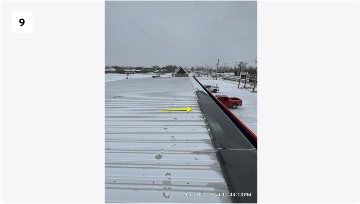
Monitor transition between roof and metal cap.
