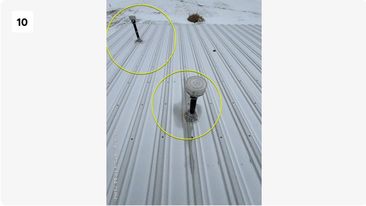
Penetrations needing tuned up and or water tested.
