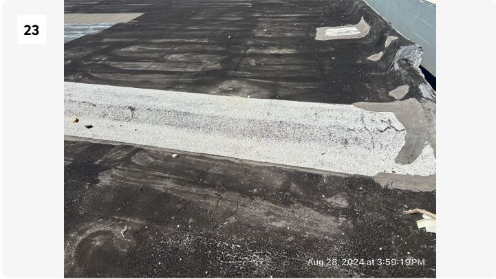
Angle changed stripped in with cap sheet. Needs to be touched up with roof cement.
