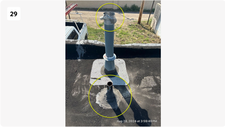
Vent cap missing and roof cement cracked out.
