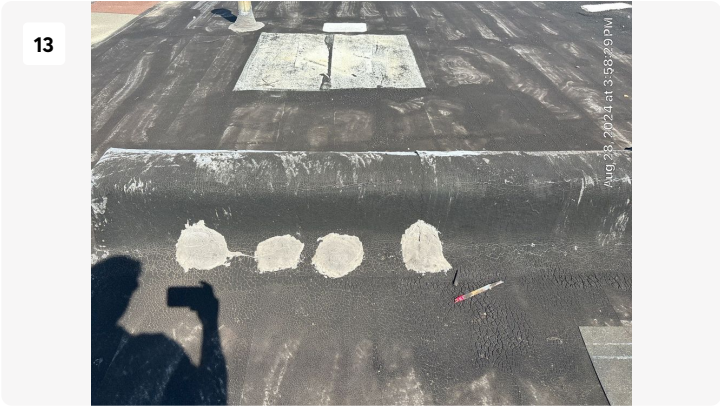
Wall flashing(s) with silicone on a BUR roof. Not the correct fix.
