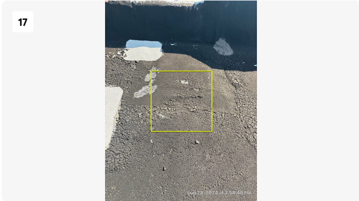
Membrane cracked out - alligating.
