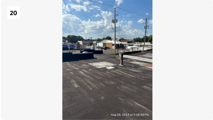
Additional photo of fiberglass and alligating.
