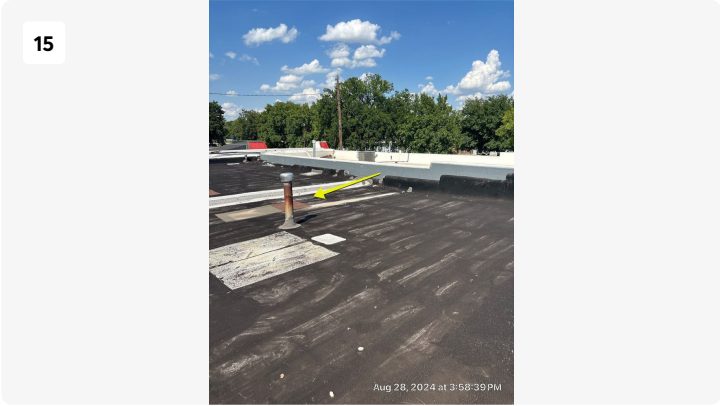
Rusted out vent cap, needs to be removed and replaced.
