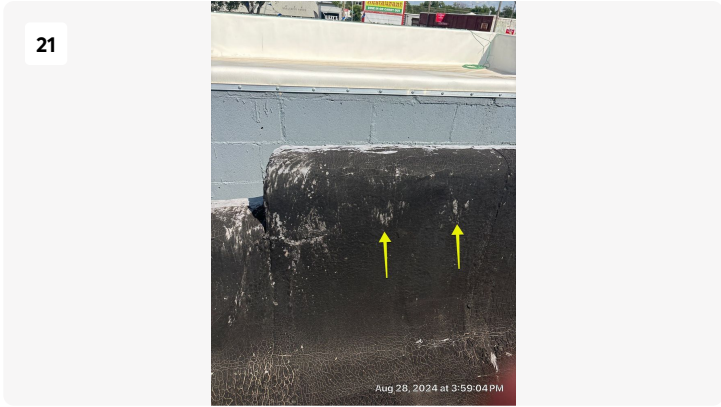
Failing wall flashing.
