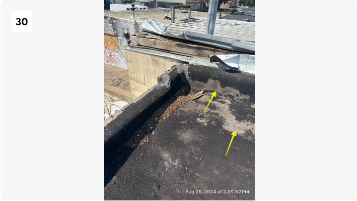
Field membrane and wall flashing both failing.
