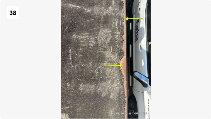
Metal edge rusted out. Needs removed, replaced and stripped in.
