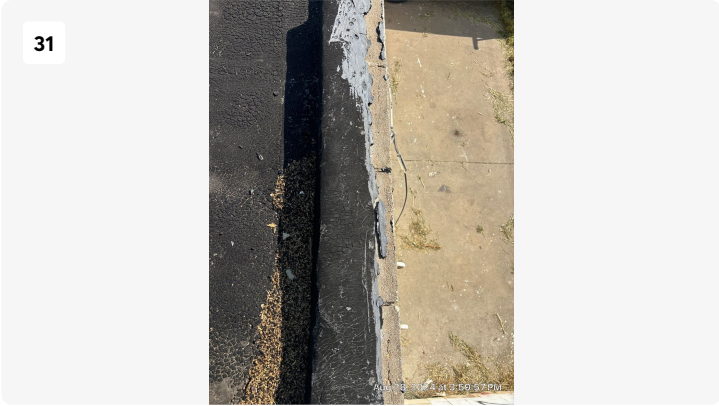
Wall termination failing.
