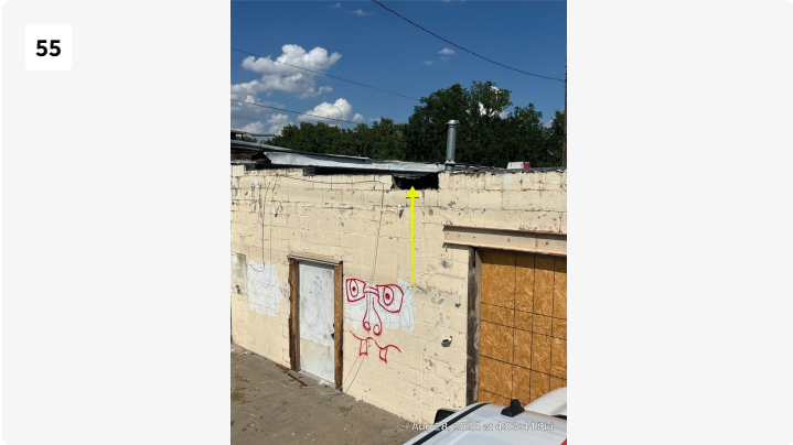
Missing masonry block.
