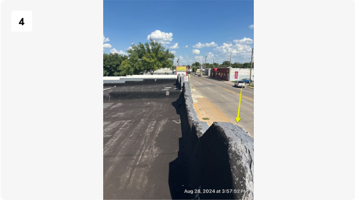
Wall termination and flashing failing. Will need new termination bar and or metal edge with new system.
