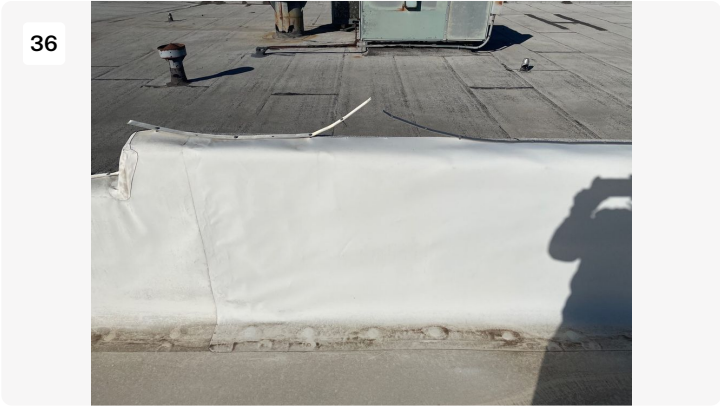
Deficiency: Termination bar completely removed from wall flashing. Project: 18492 6801 E Kellogg Date: 10/19/2022, 9:54am Creator: Evan Smith
