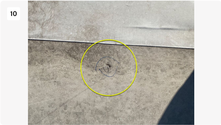
Deficiency: Open field exposure.
