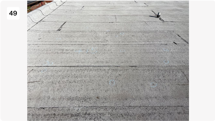
Modbitumen, mod bit roof. 15 hail hits in 10x10 square.
