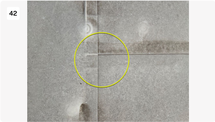
Deficiency: Missing corner.
