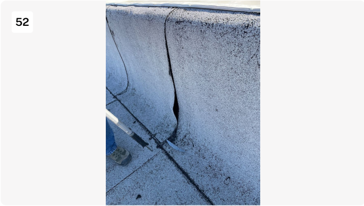
Deficiency: Loose wall flashings.
