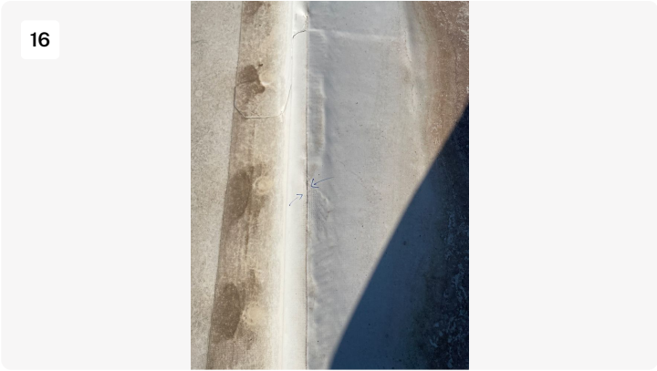
Deficiency: Missing cut edge sealant.
