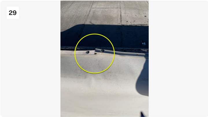
Deficiency: Termination bar fastener backing out.
