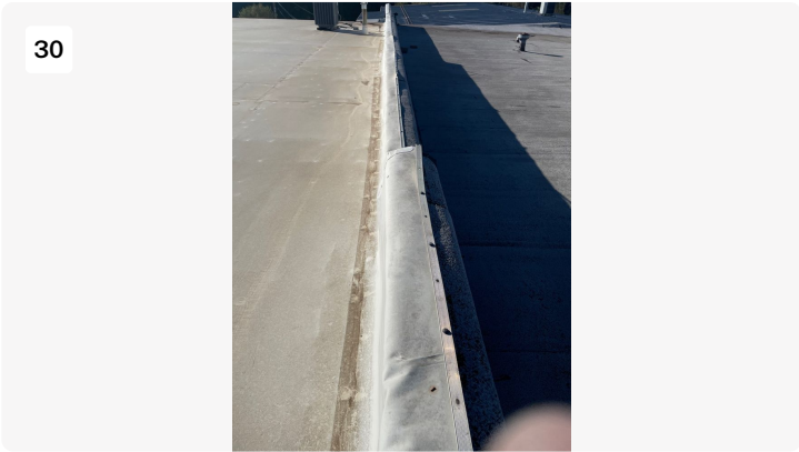
Overview of termination bar.
