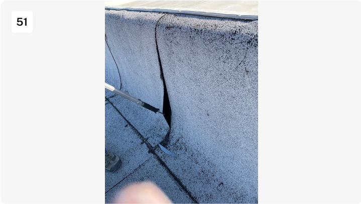
Deficiency: Loose wall flashings.
