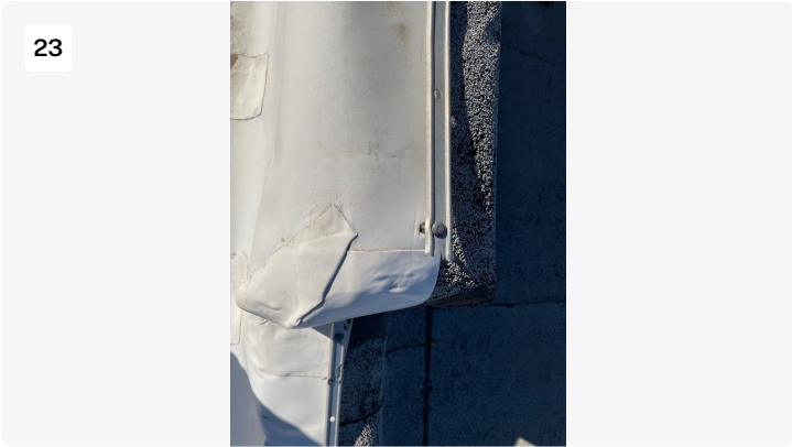
Up close on termination bar.
